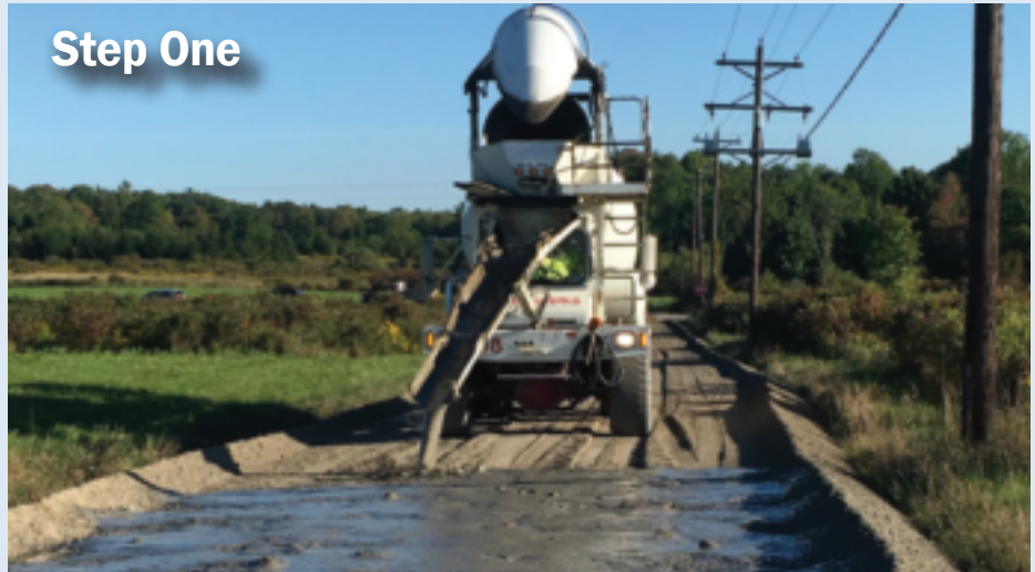
The cement slurry is distributed across a road in Lenox Township, Susquehanna County.
