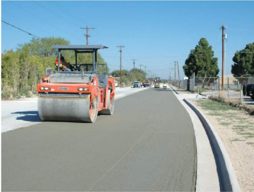
The City of San Angelo specified diamond grinding to improve rideability and increase friction. At $3 to $5/square yard, diamond grinding costs less than an asphalt overlay and produces a surface that's virtually maintenance-free. Grinding was performed by Penhall Co. Inc. of Anaheim, Calif.
