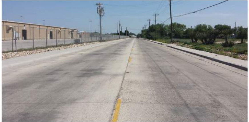
Built in 2011 by San Angelo contractor Reece Albert Inc., Texas' first publicly owned roller-compacted concrete (RCC) street is performing well, as illustrated by this photo taken in fall 2014.
