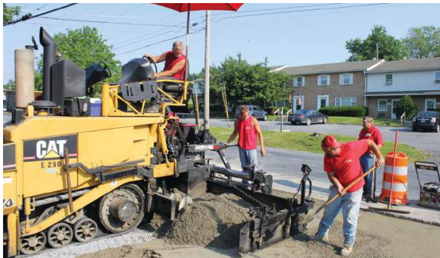
Upper Nazareth Township in Northampton County, Pa., served as a test site for roller-compacted concrete (RCC), a low-cost paving option. Applied to a 420-foot section of road that’s been in use for about two months, an official says “it looks as good as the day we finished it.” Photo: Sean Dooley, Keystone Consulting Engineers
