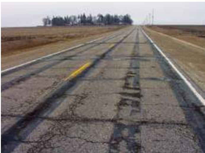
Figure 34. Poor to deteriorated asphalt pavement to be resurface (source: Todd Hanson, Iowa DOT)
