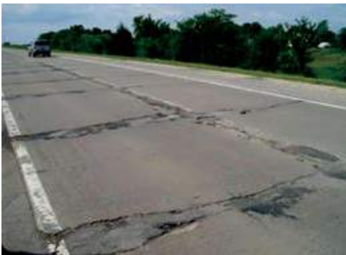
Figure 44. Route D35 existing pavement in poor condition (source: Todd LaTorella, MO/KS Chapter, ACPA)
