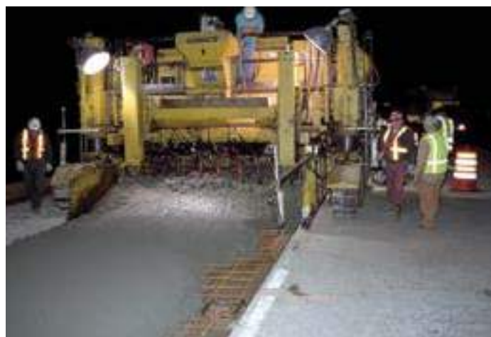
Figure 99. Controlling paving profile using a paver ski on the adjacent lane (source: Wouter Gulden, southeast chapter, ACPA)
