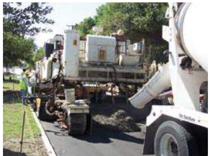
Figure 97. A typical four-track paver modified to three tracks, providing zero clearance in a C/G situation in Oklahoma (source: Jim Duit, Duit Construction Co., Inc.)
