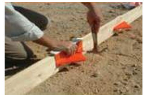
Figure 67. Taper-shaped construction joint plate dowel using fixed forms (source: Nigel Parks, PNA Construction Technology)
