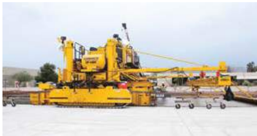
Figure 98. Controlling paving profile using a moveable stringline on the adjacent lane (source; Kevin Klein, Gomaco)
