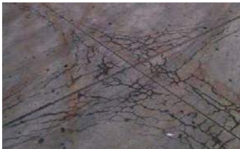
Figure 10. Moderate ASR cracking along the perimeter of slabs (source: [Thomas et al. 2011])
