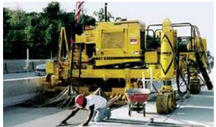
Figure 96. A three-track, zero-clearance paver placing concrete along a median barrier (source: Kevin Klein, Gomaco)
