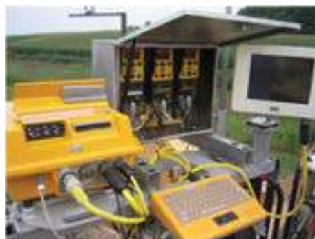
Figure 143. GPS paver control system
