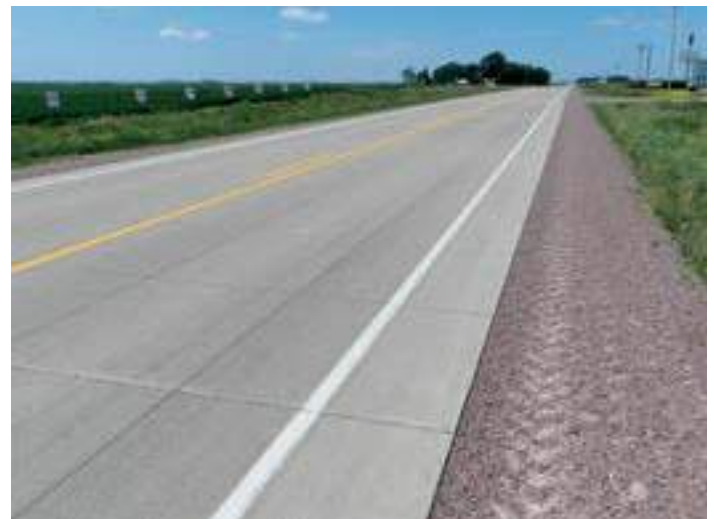
Figure 35. Poor to deteriorated asphalt pavement resurfaced with unbonded concrete overlay (source: Kevin Merryman, Iowa DOT)
