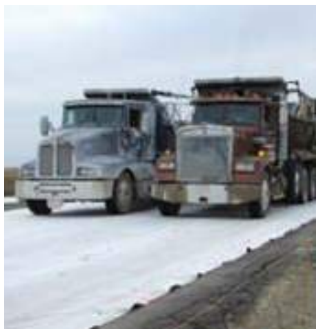
Figure 113. Paving on top of white geotextile fabric interlayer (source: Larry Engbrecht, South Dakota chapter, ACPA)
