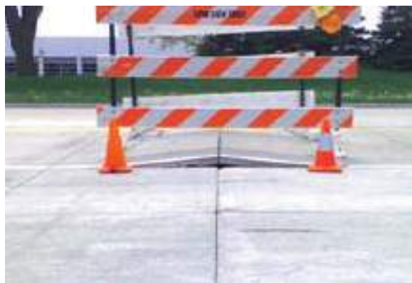
Figure 52. Overlay blowup where expansion joint should have been cut over existing concrete expansion joint (source: Dan DeGraaf, Michigan Concrete Paving Association)
