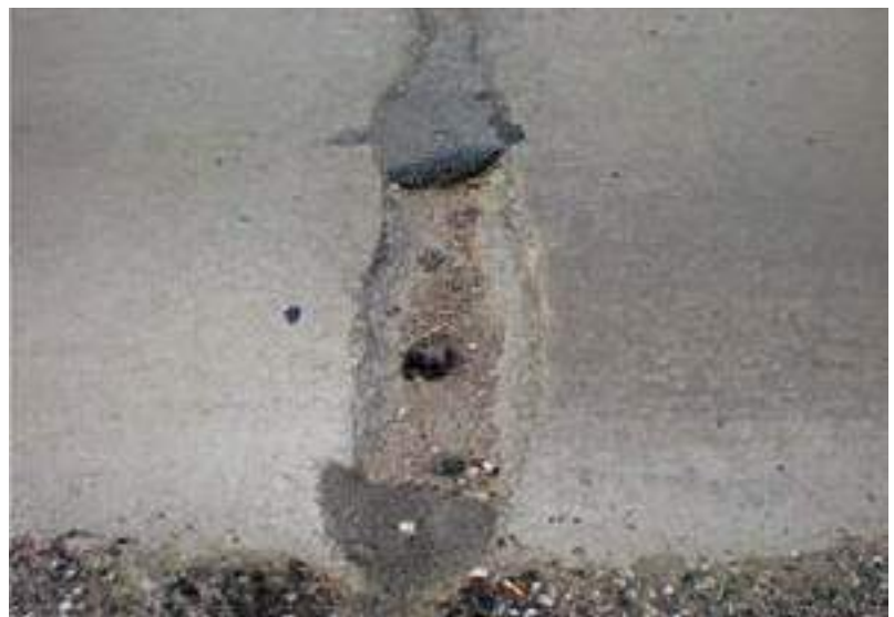
Figure 12. Typical joint deterioration with HMA patch (source: Trinity Construction Management Services, Inc.)
