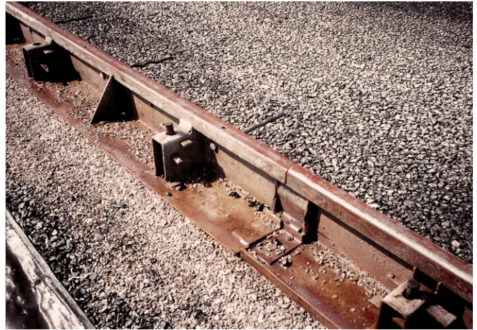
Figure 10. Forms should rest on a level surface, and should be fastened securely and pinned in place.
