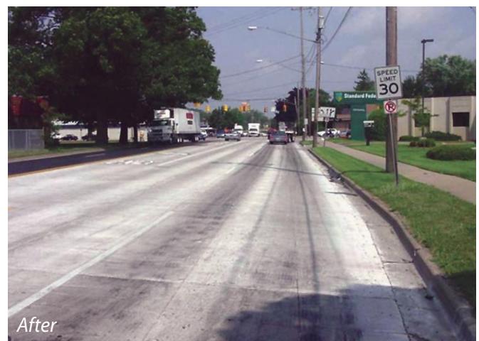
Figure 2. These before (top) and after images show a concrete inlay extending well beyond the physical area of an intersection in Western Michigan.
