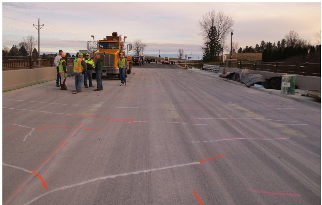
Figure 1. Cracking (marked on deck surface) occurred before this newly constructed bridge was opened to traffic.
